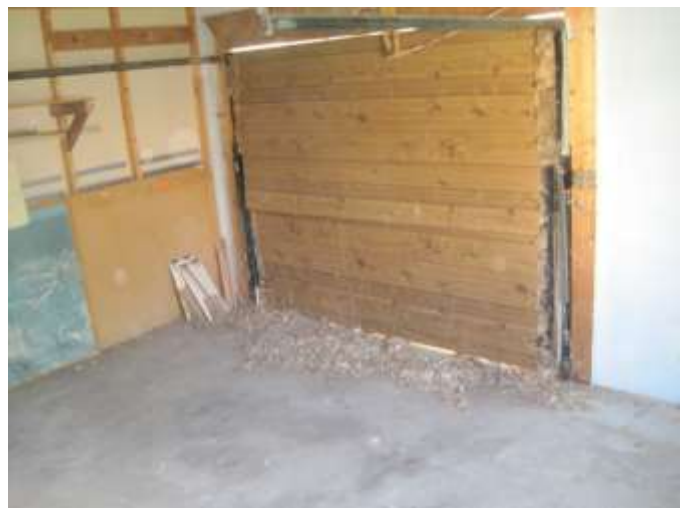
Rear of building has been walled off and had a garage door
