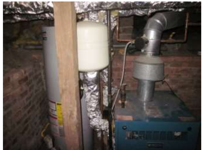
40-gallon natural gas water heater, Hot water system for radiators
