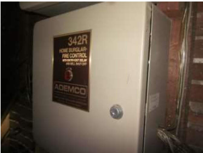
Burglar & fire alarm system panel
